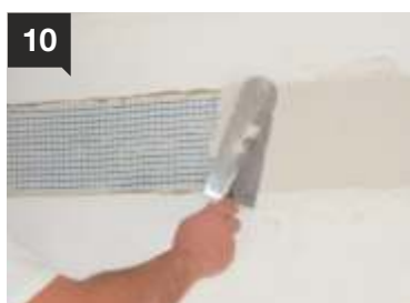
10 After the first layer has dried, the surface is dampened and the second layer of UNICRET or UNICRET-FAST is applied.
