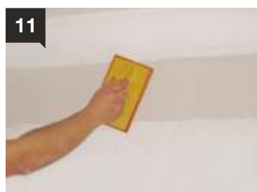
11 After the plaster has slightly dried, it is rubbed with a sponge faced-float.
