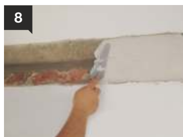
8 A first coat of plaster is applied, using UNICRET or UNICRET-FAST , improved with ADIPLAST polymer latex.
