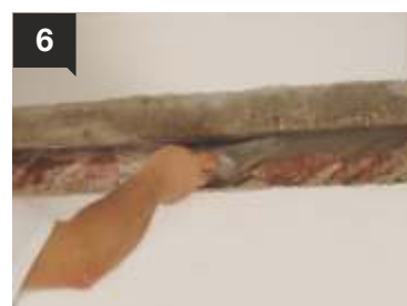
6 Finally, DUROCRET , DUROCRET-FAST or RAPICRET may fill the widened crack, as deep as possible, using a gauging trowel.
