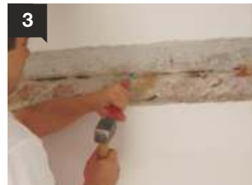
3 Then, the area of the detachment is widened by breaking the surrounding bricks with a sharp tool.
