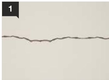
1 A cracked or detached masonry results in cracks on plaster.
