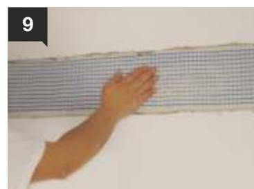
9 While the first coat is still fresh, a strip of fiber-glass mesh is placed and is slightly pressed onto the first coat.
