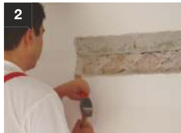
2 Firstly, the plaster is removed to a total width of 30 cm (15 cm on each side) along the entire length of the detachment.
